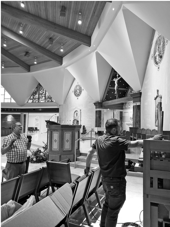
Technicians with the Buzard Organ Company of Champaign, Illinois, work on voicing pipes for the new organ that’s being built for the Cathedral of St. Joseph in Jefferson City. The new organ, part of a comprehensive renovation of the Cathedral, is slated to be installed in early 2024.
